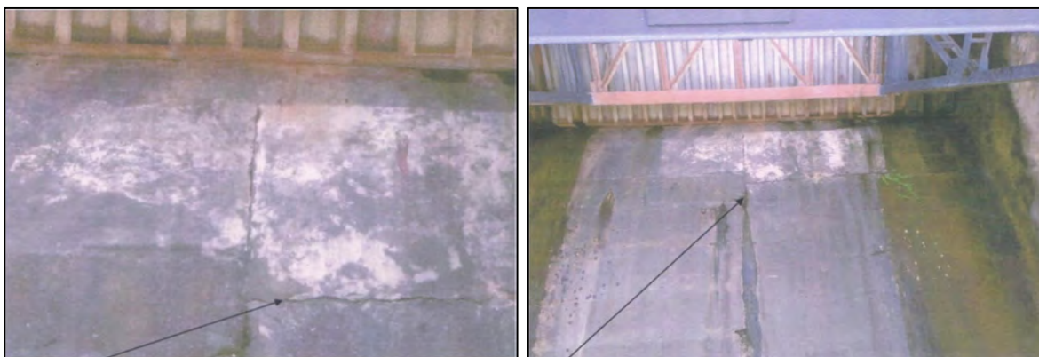
Crack & Leakage seen in Glacis Portion
