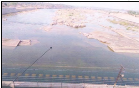
Damaged Portion of End Sill
