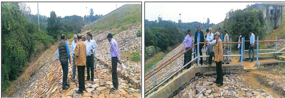
Disturbed u/s rip–rap/ pitching
