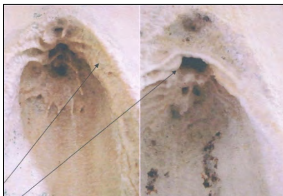
Choked Drain in Gallery
